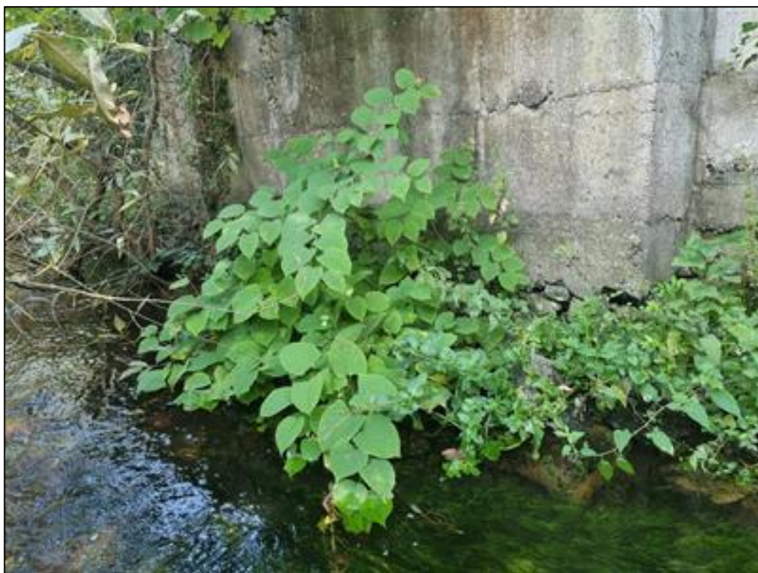
Plate 3-7 Japanese knotweed at the bottom of the embankment of the Gaol River to the north of the McLaughlin Building
